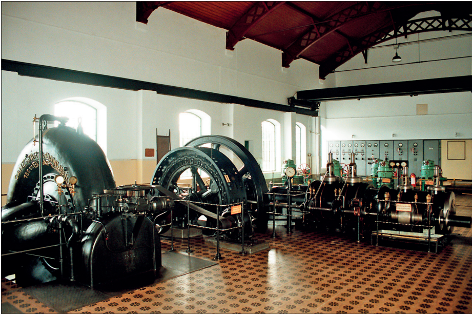
Pic. Nr. 3: László Péchy Flood Gate and Pump Station, Nagyecséd. 2022.
