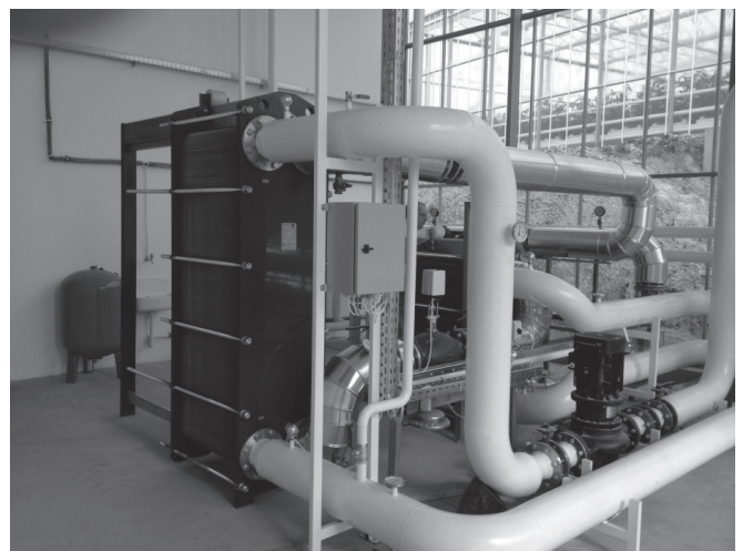
Figure 4: Sheet-metal heat exchanger used at the first heating cycle
