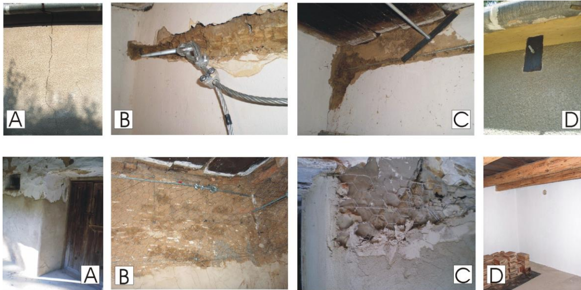
Figure 10. Two renovation processes of the adobe house. Upper part: strengthening of the upper part of the walling: (A) splitting (B) connection of the cable-roping to the screw (C) The stretched cable-roping in inside (D) The screw with underlay in outside. Lower part: Strengthening of the surface: (A) the moulding surface in outside (B) the wire mesh mounted on the wall (C) rough-casting (D) polished plastering in inside. (Source: Experimental work by the first author)
