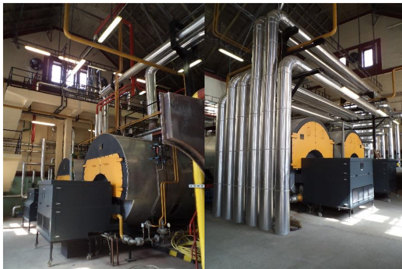
Figure 1: AKH-4/12 steam boilers (left side) and AKH 7500M hot water boilers (right side)
