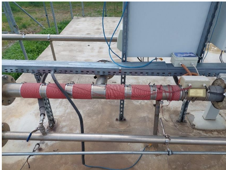
Figure 4. Electromagnetic system protecting the stainless-steel pipeline section leading to the degasifier (Nagyszénás)
