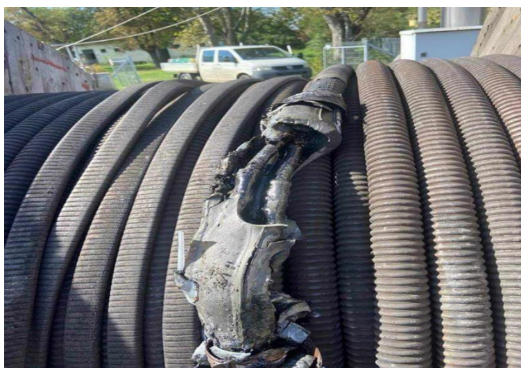
Figure 2. Insulation damage to the thermal water pump's electrical cable (Nagyszénás)
